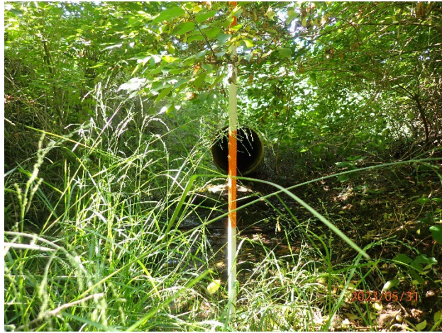
Embankment drain pipe outlet- note excess woody vegetation to cut and remove
