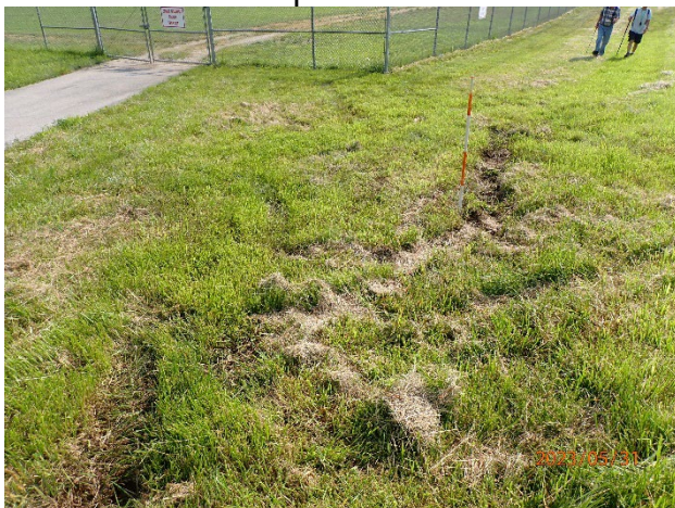
Seepage area at toe and left groin
