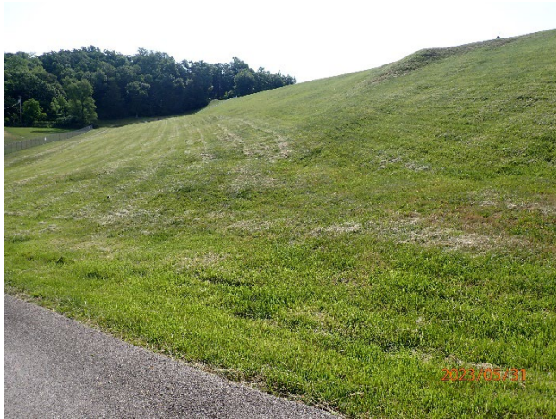
Downstream face- note historic bulge/uneven surface to monitor for change/movement
